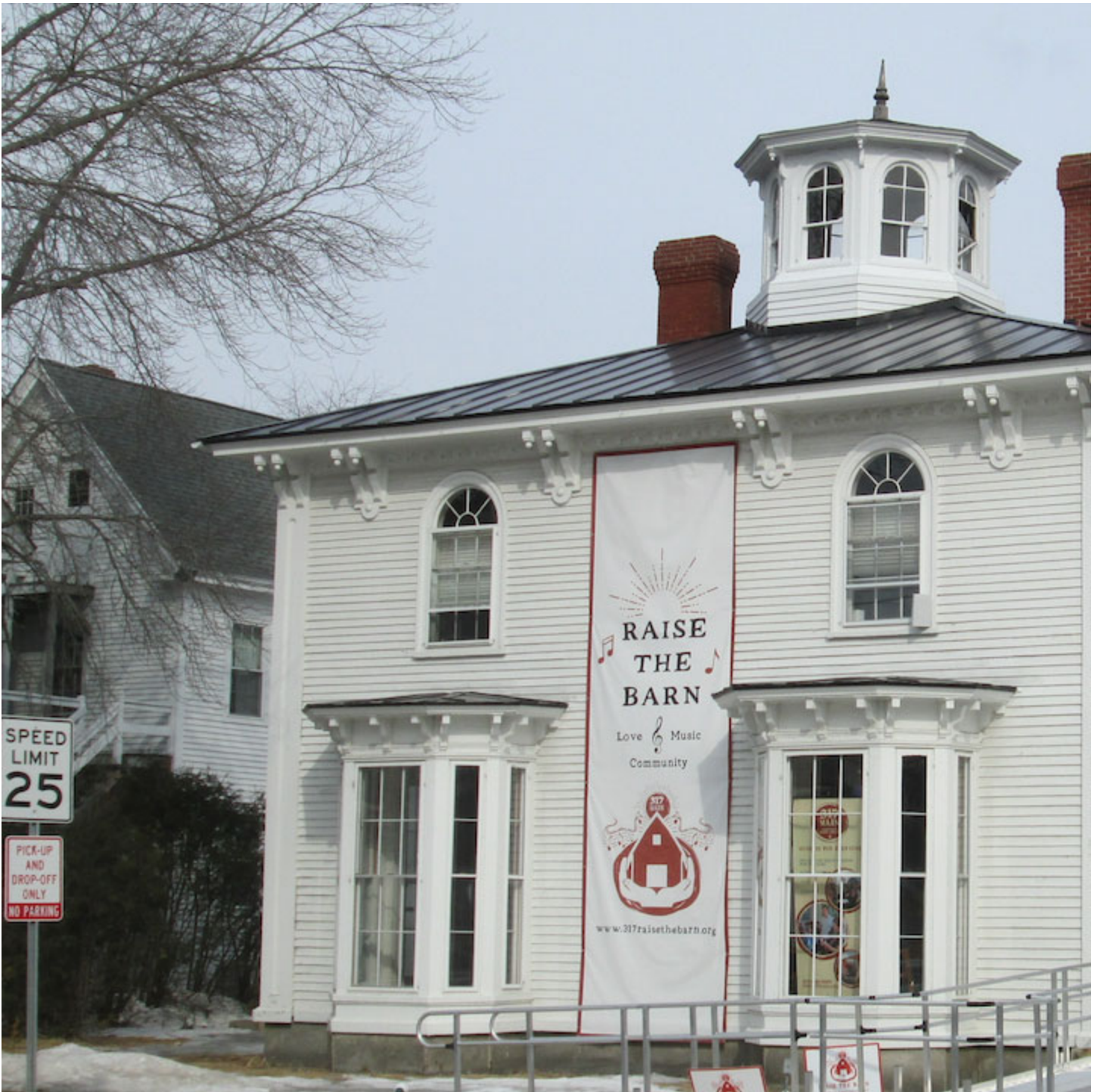
The entry way to the house has obviously been replaced at some point in the Victorian Era, see the Italianate brackets supporting the entry hood, which appears to be in need of work. These changes are authentic, not of an uncommon type, and could well be retained.
