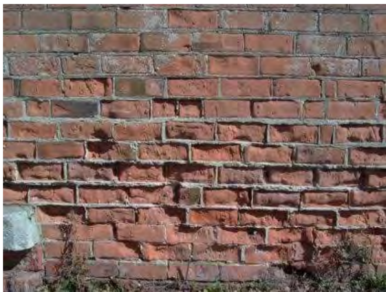
An example of how the wrong mortar mixture was too strong and caused irreparable damage to the historic brick.
