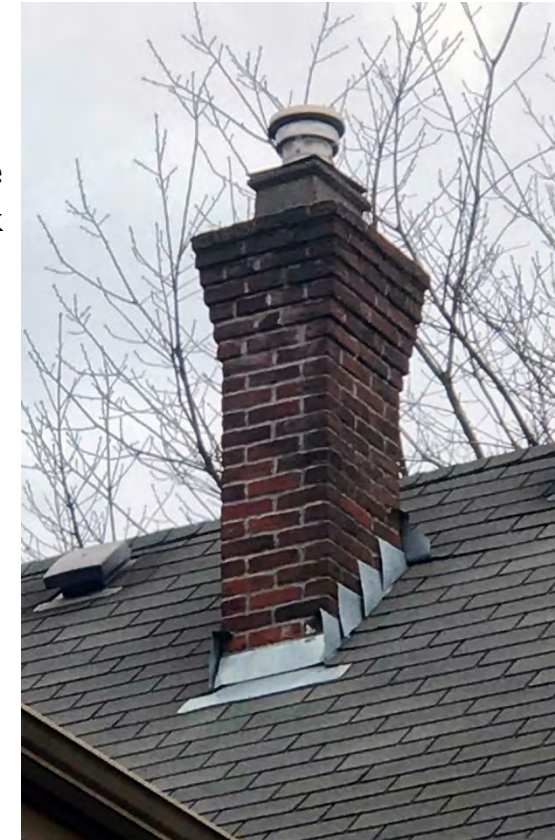
Improper modern chimney cap
