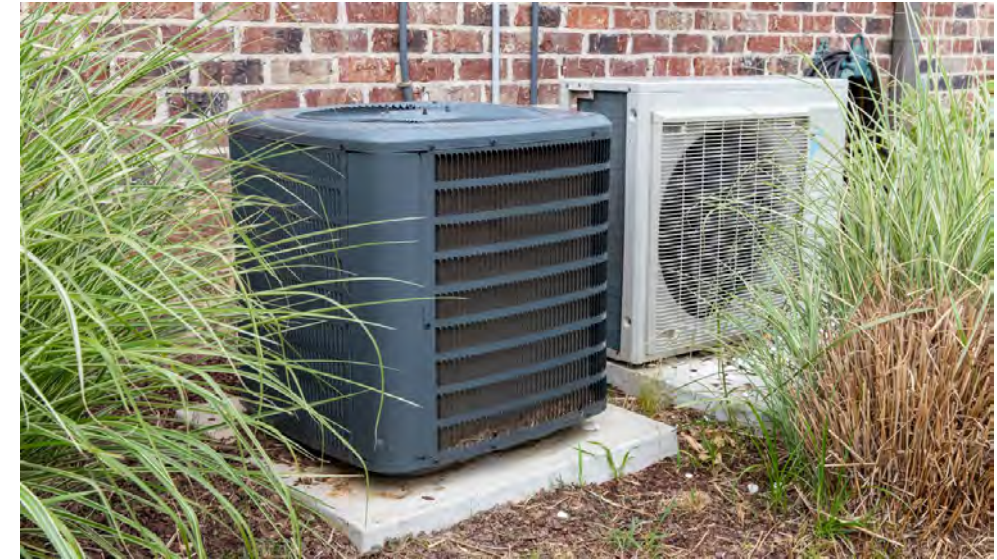
Mechanical equipment should be screened with vegetation, and installed where not visible from the public street.
