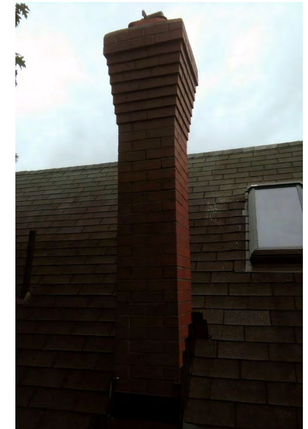
New, low profile chimney cap
