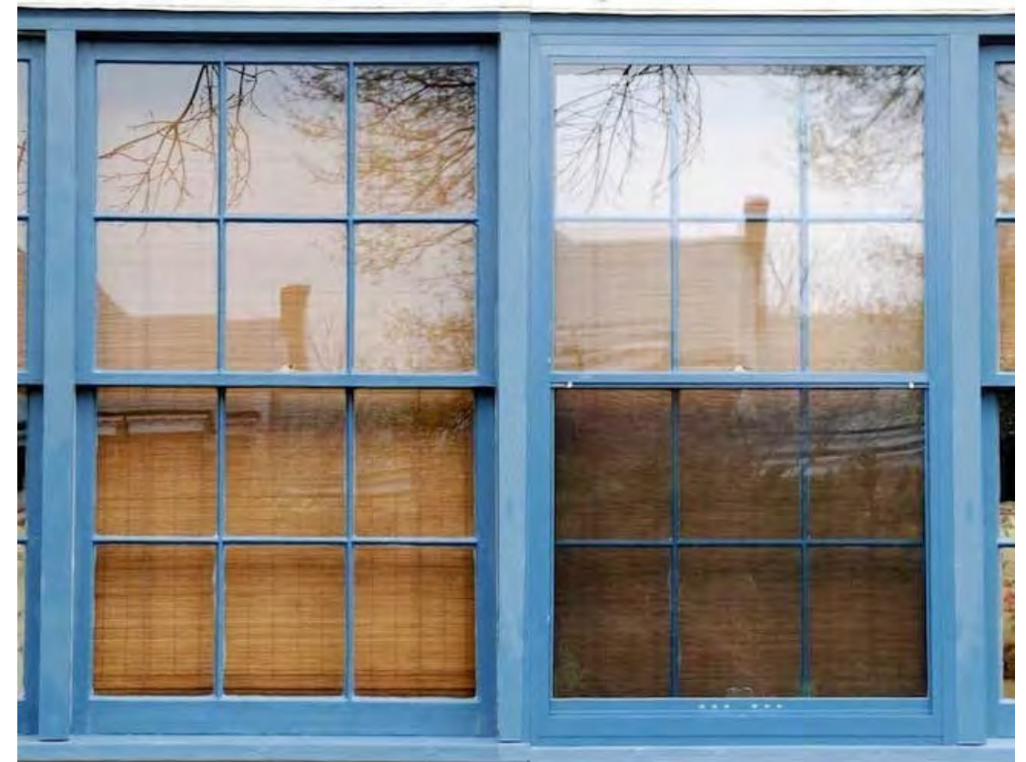
An example of good exterior storm windows installation. Storm windows can increase energy efficiency of a building, without losing historic fabric or visual character.
