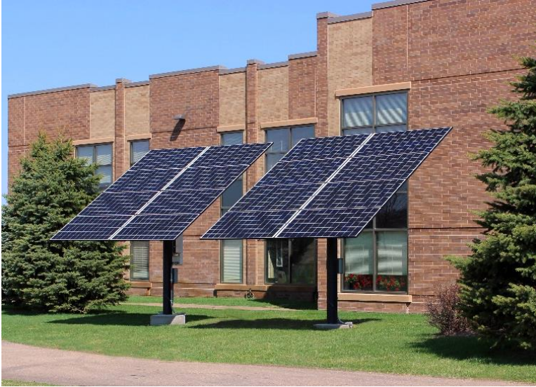
Minnesota Municipal Power Agency 5 kW Hometown Solar Shakopee, MN
