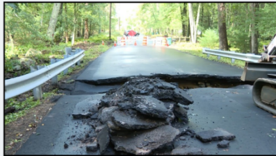
Excessive Flooding Caused Brandy Brook Road Failure (September 2023)
