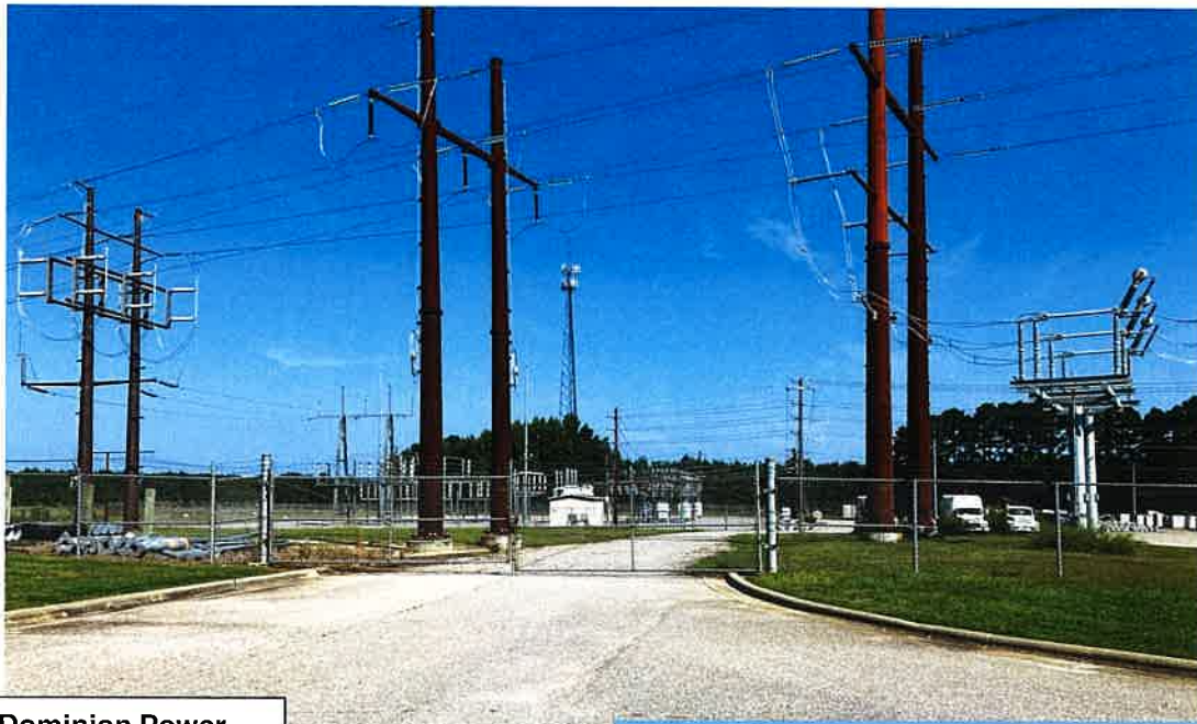
Dominion Power Tarboro Sub-station
