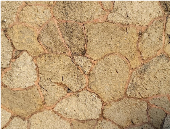
Figure 10: Polygonal masonry formation, where each coquina rock was cut into organic, natural shapes and fit together.
