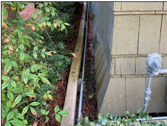
Figure 6: Close up of sloped siding at foundation and concrete band that follows the foundation.
