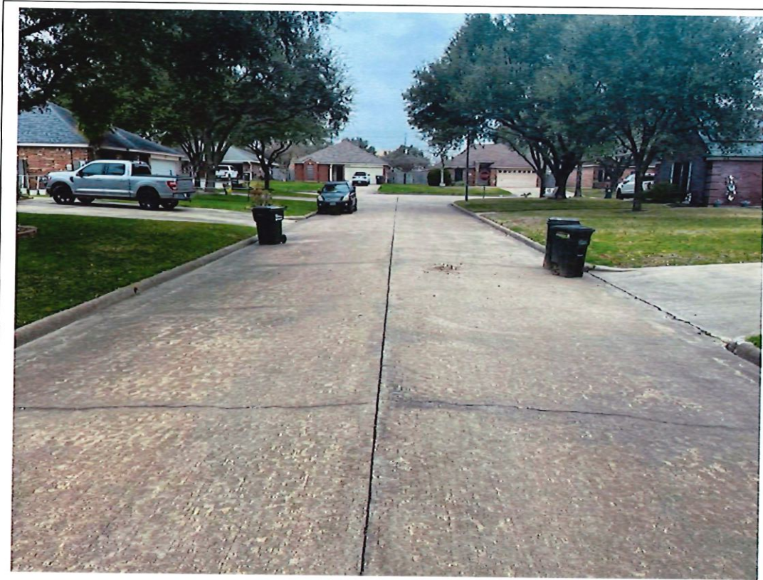
Figure 4 Shadowlake Court–Regular Unsealed Tight Transverse Cracks
