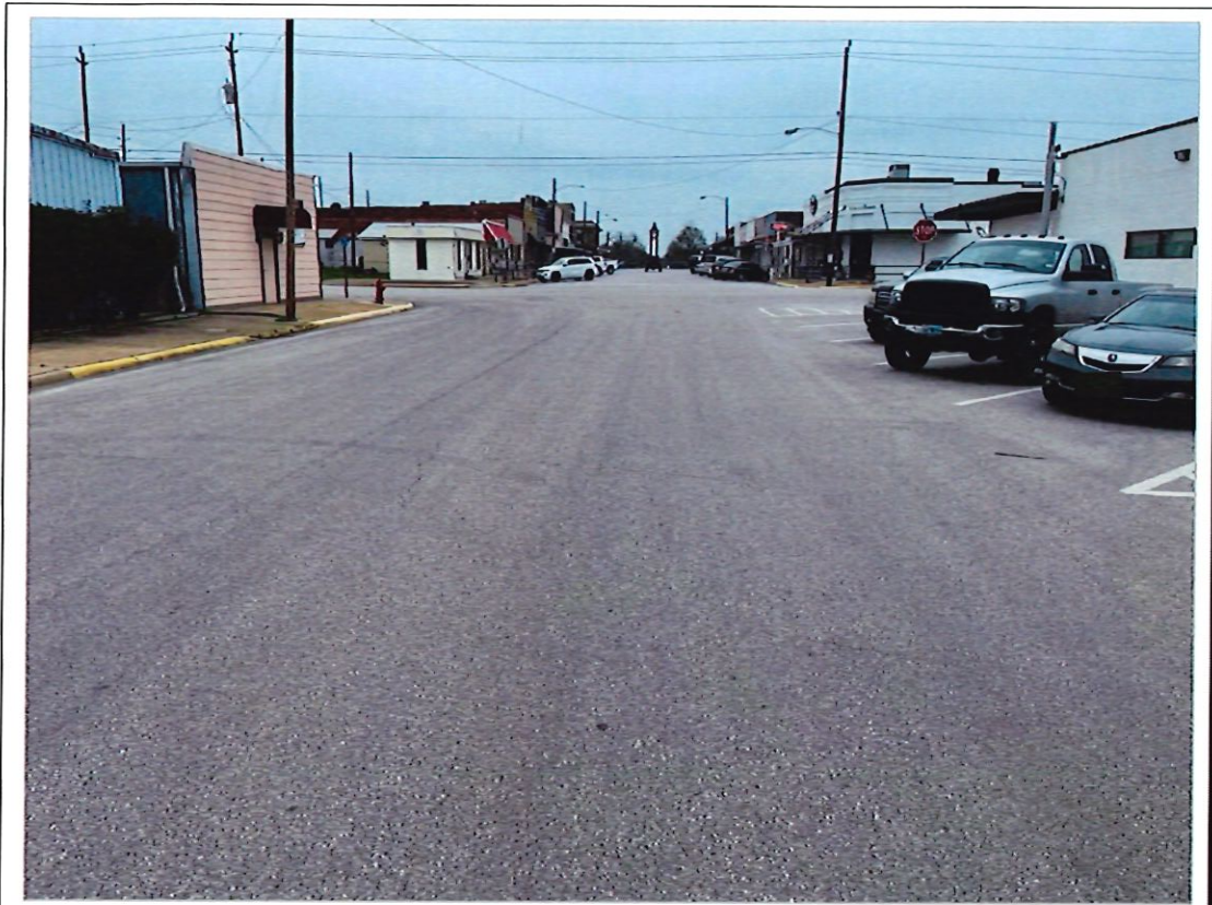
Figure 2 Fowlkes Street–Light Surface Material Raveling
