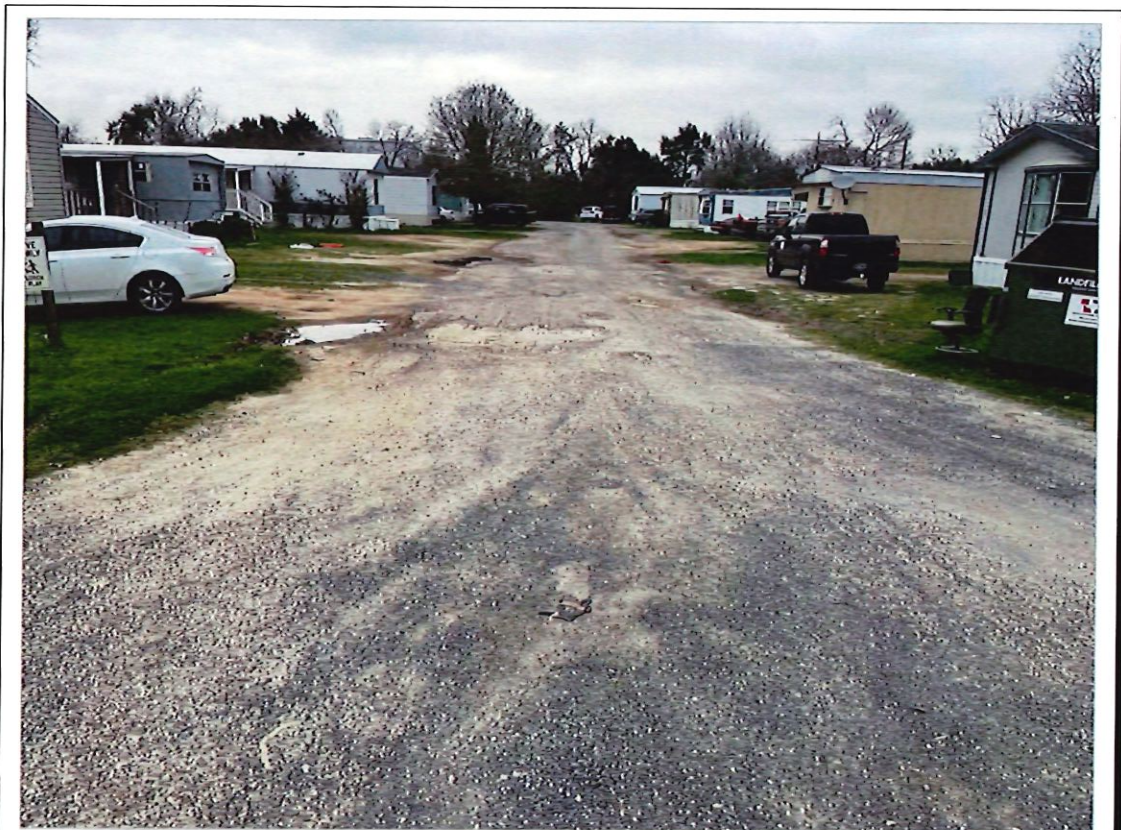
Figure 8 Lux Street–Severe Raveling, Loss of Surface Integrity, and Potholes
