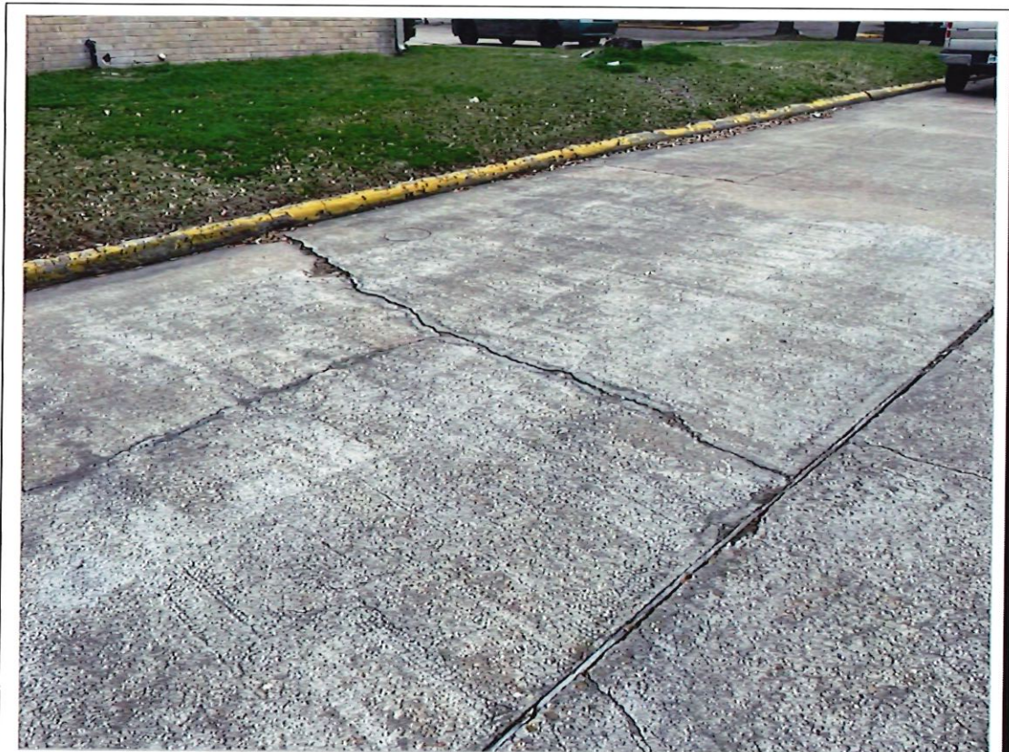
Figure 7 Vail Street–Open and Spalled Joints, Moderate Block Cracking
