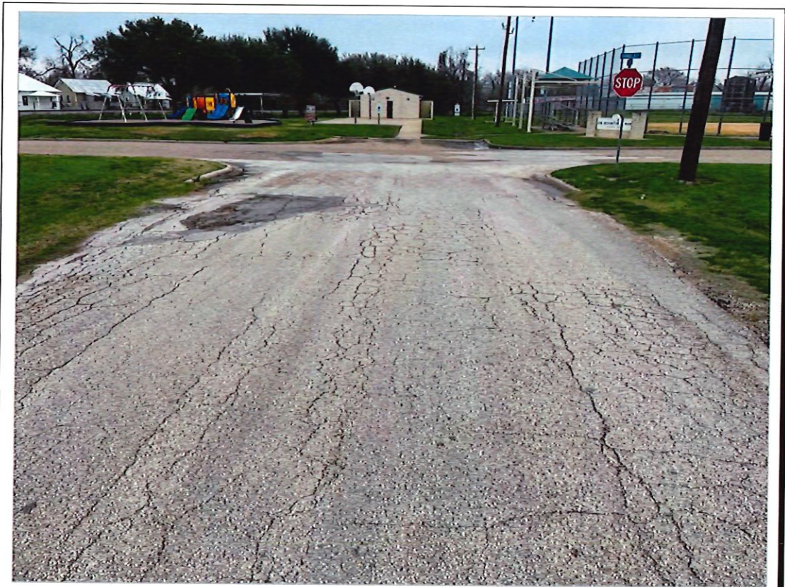
Figure 6 East 2nd Street–Severe Alligator Cracking
