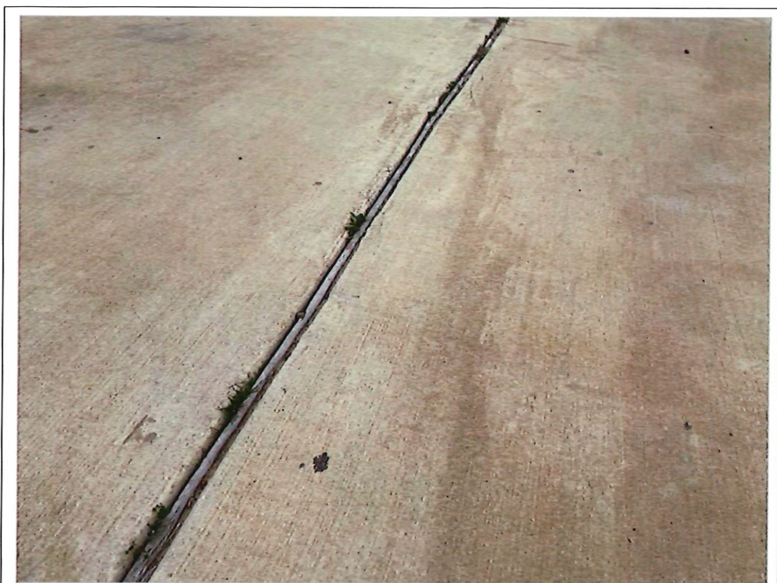
Figure 3 Mourning Dove Drive—Unsealed Expansion Joints
