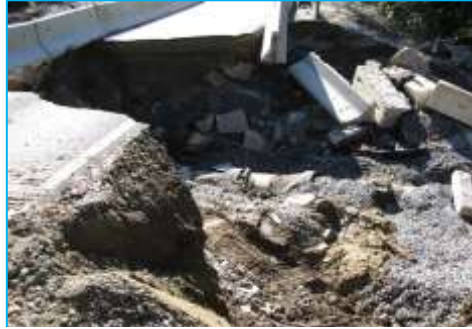
Depot Road Culvert Failure, September 2008
