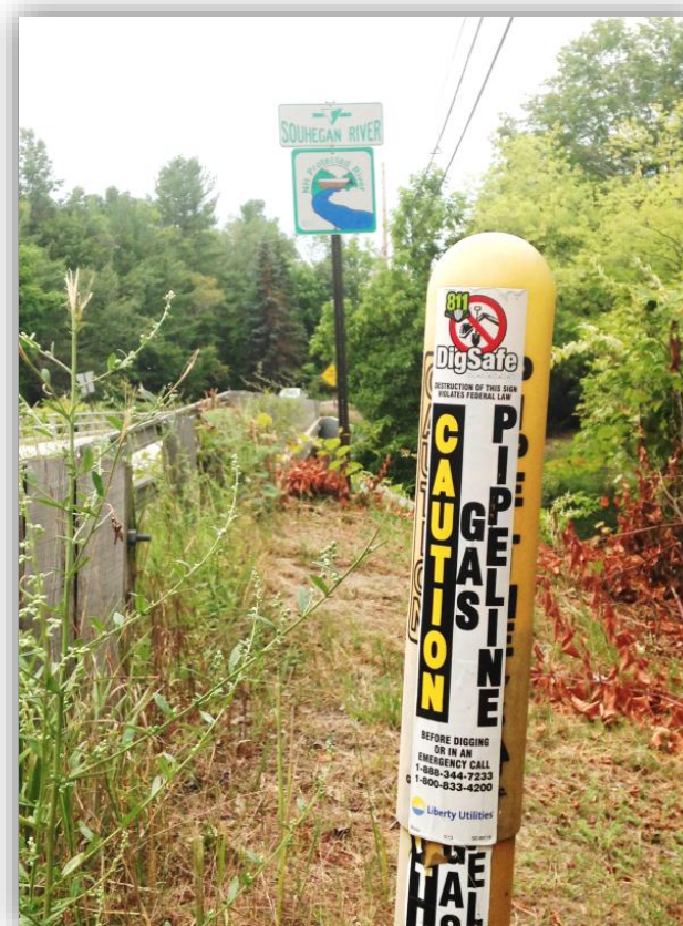
Gas line marker along the Souhegan River, Merrimack, NH. Image source: NRPC.
