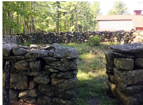
The partially restored remnant of the Wilton Town Pound Image Credit: Wilton Planning Board & NRPC
