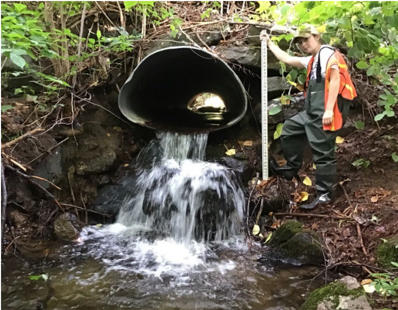
Figure 16. Perched Culvert in Milford. Credit: Stream Crossing Initiative, 2021.
