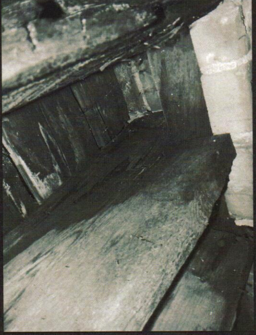
Roof rafter & sheathing failure
