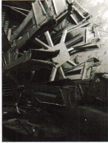
Damaged Roof Lantern
