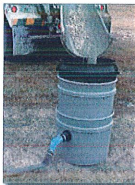
Figure 3. Concrete washout filter
