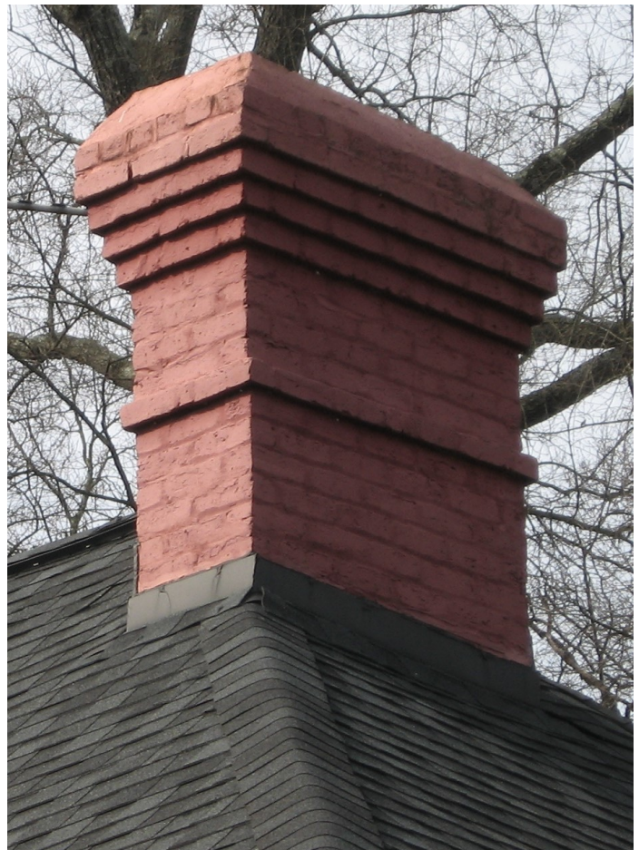
Corbelled brick chimneys are distinctive architectural features that add to the historic character of a dwelling.
