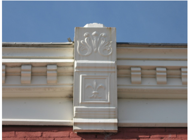
Upper façade features may include sheet metal cornices (above, or other features such as parapets and finials (bottom).
