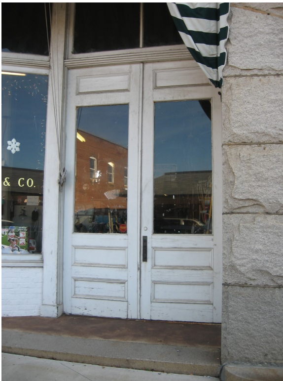
These double doors and transom are remarkably well preserved and are significant features to this building.
