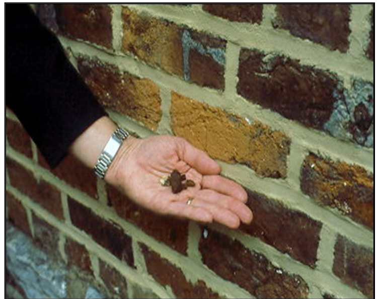
Over time, poor repointing and abrasive cleaning can lead to sections of the brick wall deteriorating.
