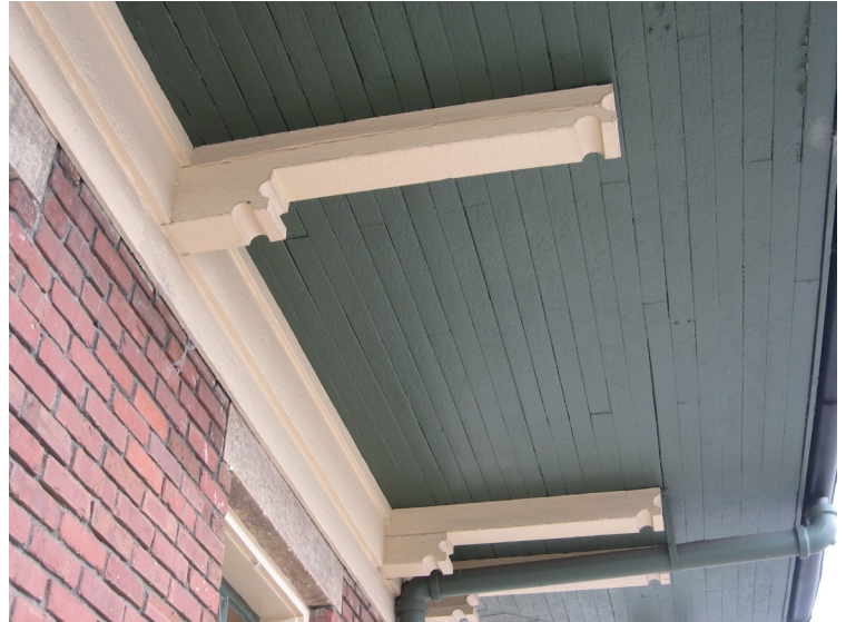
Wood elements such as these rafter ends called purlins are used on the train station.
