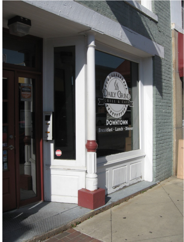
This original cast iron column is an important feature on the storefront.
