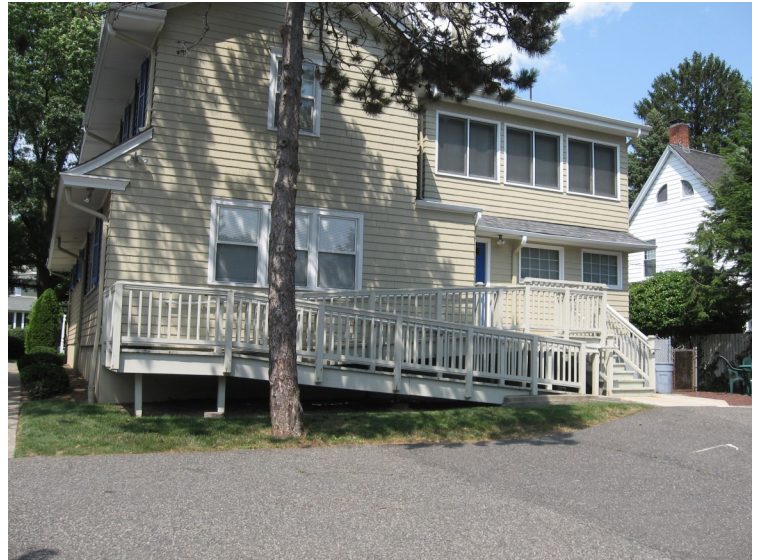
ADA compliant ramps should be located at rear elevations and where there is a dedicated handicapped parking space.
