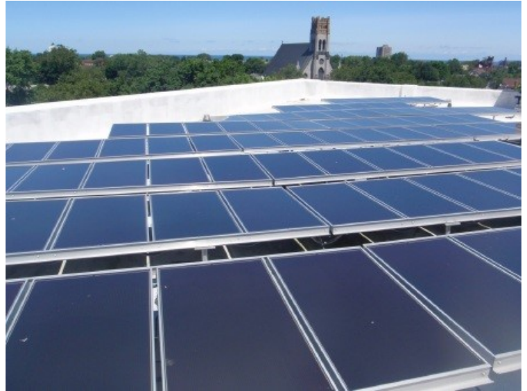
The installation of solar panels on roofs of commercial buildings is appropriate and encouraged. These panels shall be sited below a building's parapet wall and not visible from the street as shown in this example.
