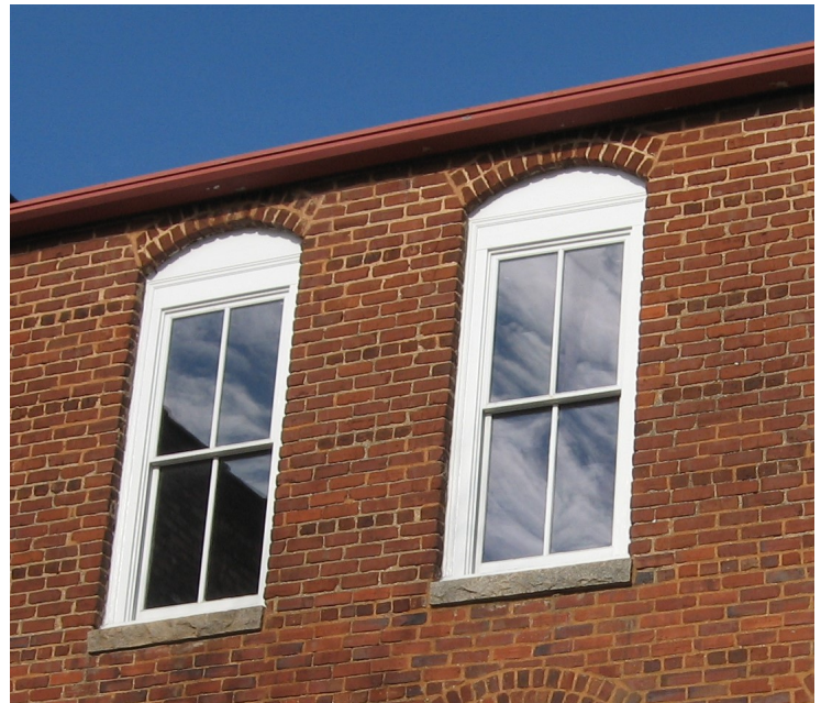
These replacement windows correctly fit the opening, have true divided lights, and accurately resemble historic wood sash designs.
