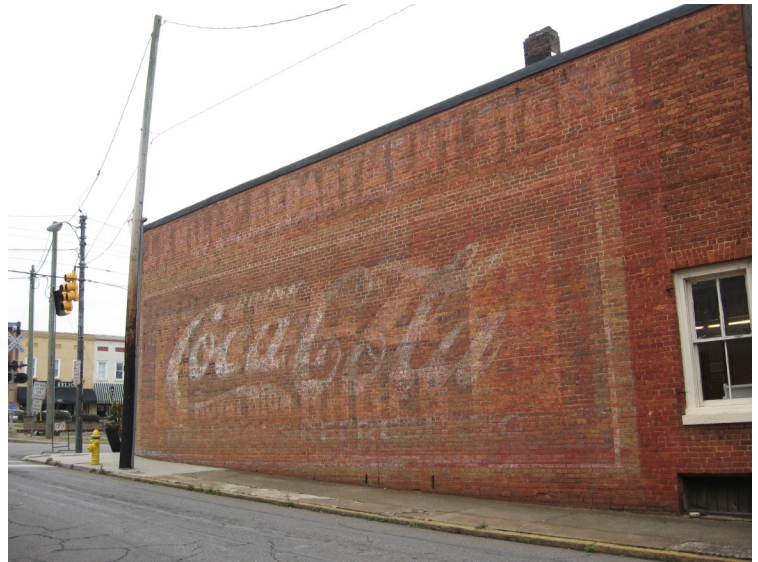
Historic “ghost” wall signs should be restored rather than painted over with new murals. .
