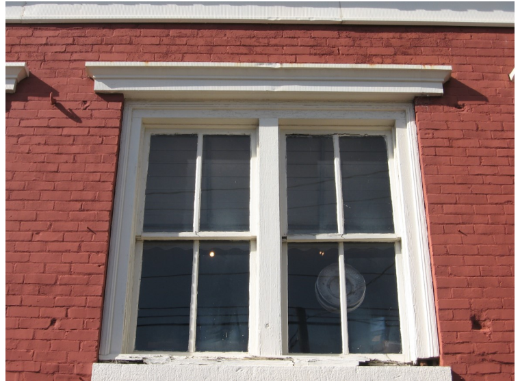
Preserve original windows and components like this pair of two-over-two, wood-sash windows and wood lintel.
