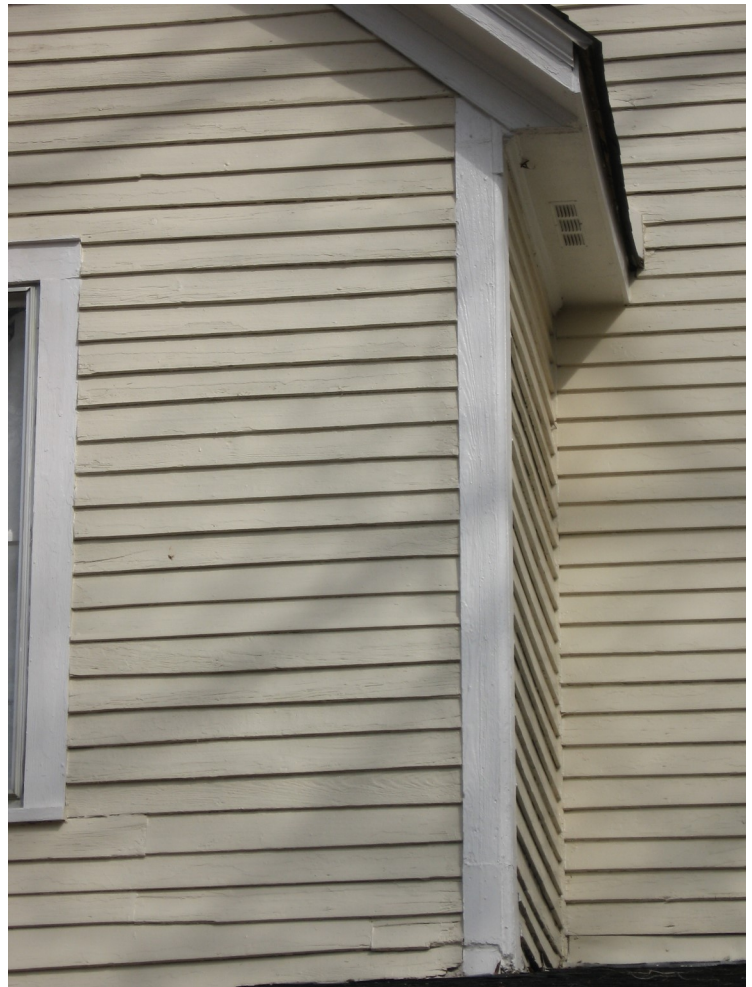
The original weatherboard siding contributes to the historic character of the building.
