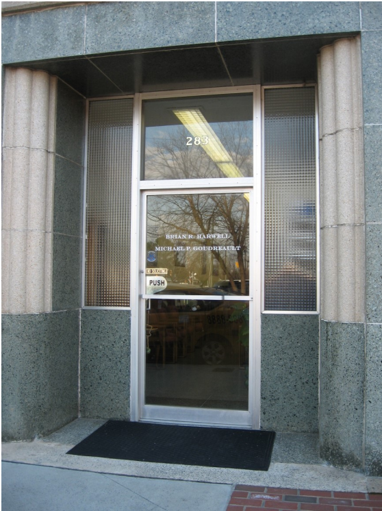
This ca. 1945 entrance has a glass and metal door with textured sidelights that help define the style and period of the building.
