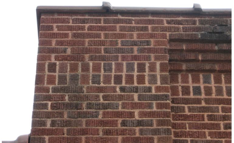
Preserve and maintain original masonry walls such as this textured and varied colored brick.
