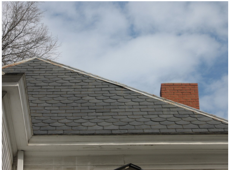
Original slate roofs contribute to the historic character of a dwelling and should be preserved .
