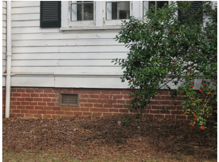
Brick foundations should be kept in good repair to ensure the longevity of the dwelling it supports.
