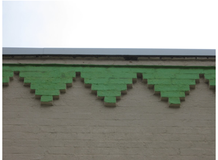
Masonry details such as corbelled brickwork are found throughout the downtown area.
