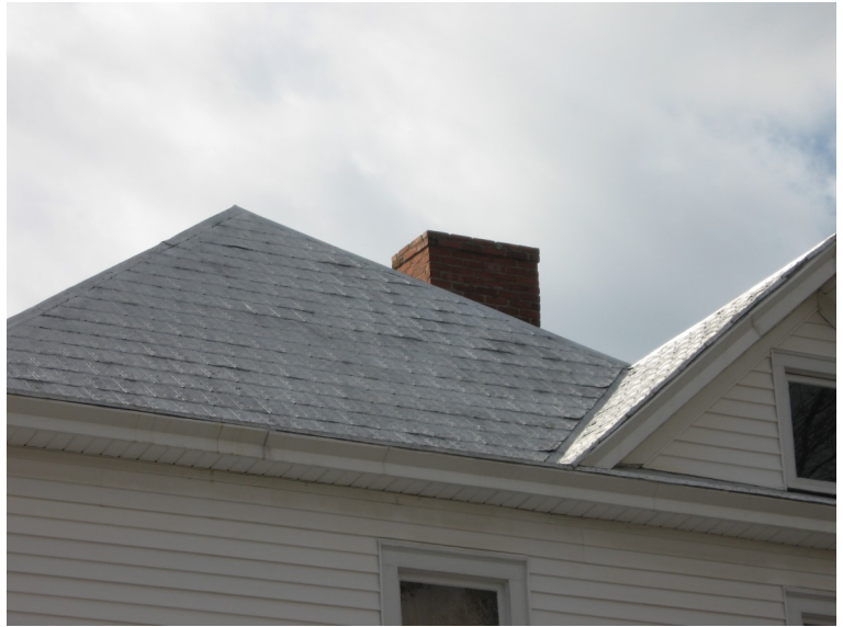
Retain and preserve original roofing materials such as this pressed metal shingle roof.
