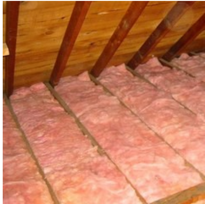
Adding ceiling insulation is one of the most cost effective methods of saving energy in commercial buildings.
