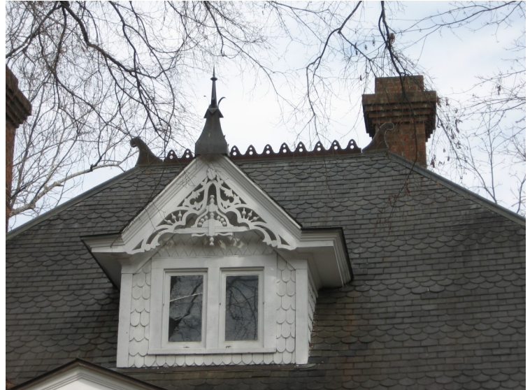
This slate roof features a unique pattern of square and scalloped tile, metal crest work, and a decorative finial.
