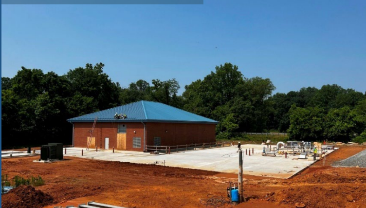
Wiggins Road Pump Station
