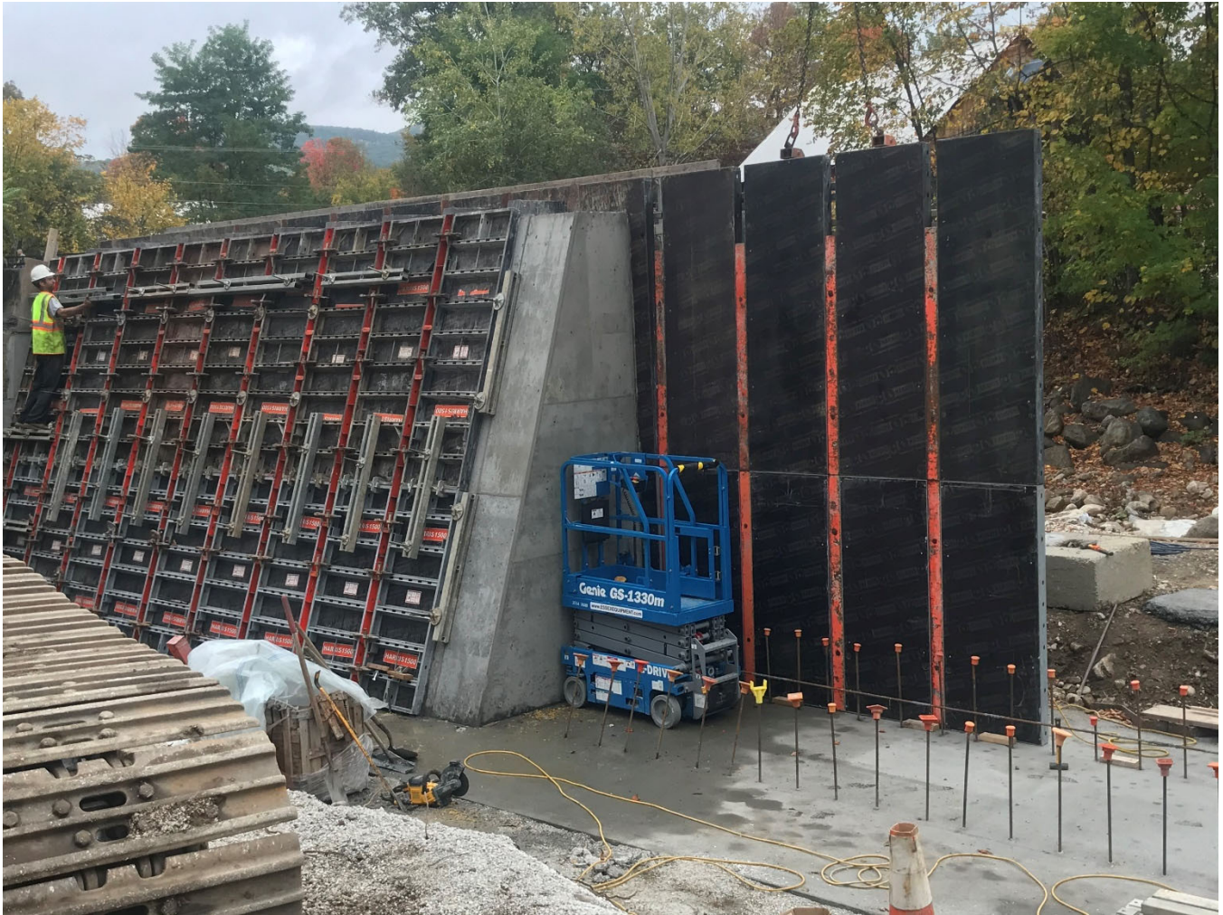
Figure 1: First section of flood wall. Form on end removed to connect to back of next section that has small offset. Front form being installed.
