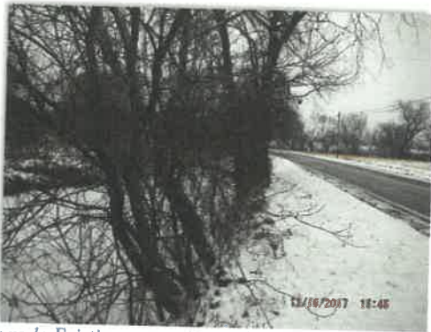
Figure 1: Existing vegetation undermined along west side of Shard Villa Road
