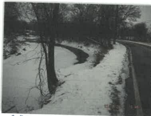
Figure 2: Pavement box-cut repairs due to close proximity of river and undermined soils beneath Shard Villa Road
