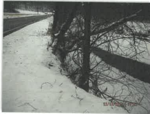
Figure 5: View of undermined bank looking south along Shard Villa Road
