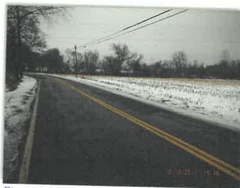
Figure 4: Closer look at recent pavement repairs
