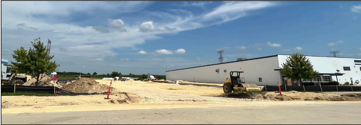
Future Site of the ABC Supply Sales & Distribution Center in Machesney Park Photo credit: Village of Machesney Park
