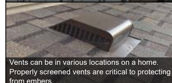
Ensure eaves are enclosed and properly maintained. The underside of eaves should be clear of any vegetation that may be growing under or near this area of the house.
