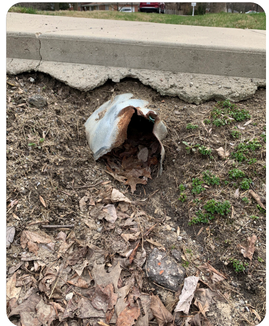
Damaged storm sewer culvert (Giffels Webster, 2020)
