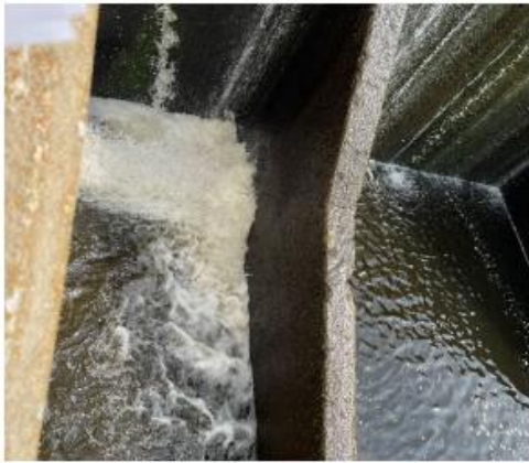
Right Buttress No apparent change in spalling.
