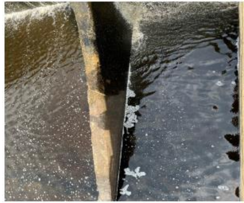
Left Buttress No apparent change in spalling.
