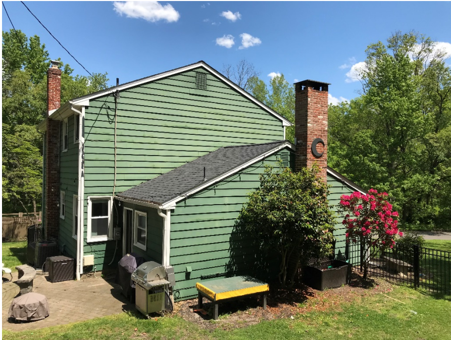
View of existing 1-story addition to be removed and replaced with a 2-story addition.
