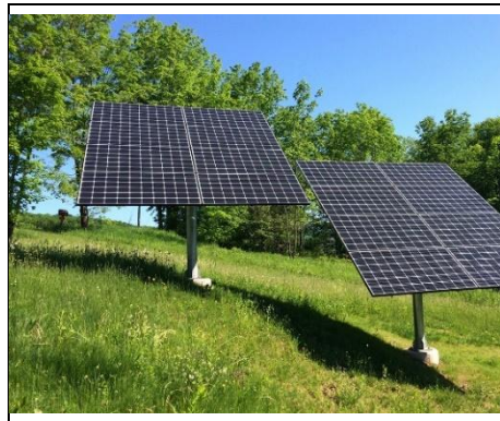
Ground Mounted Solar
