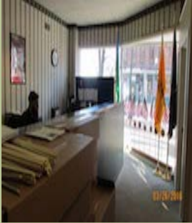
There is no interior accessible route upon entrance to the Veteran's Center.
