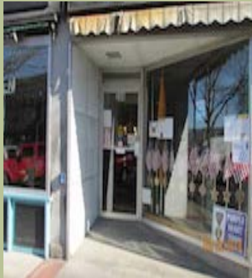
Accessible route from parking to entrance at the Veteran's Center has large crevices and is uneven.
