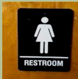
Accessible women's restrooms have non-compliant signage at Four Corners School.
