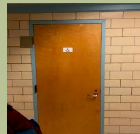
Handicap Accessible restroom in North Parish School does not have correct signage.
