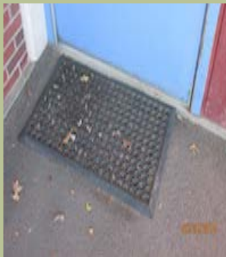
Route to City Offices entrance is uneven, damaged, and door is not ADA compliant.
