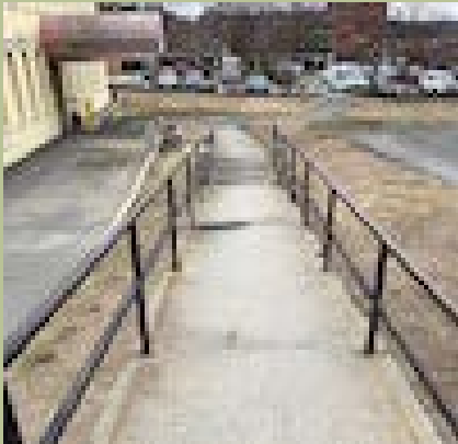
The library's accessible entrance ramp has cracks and crevices. Route from parking to entrance crosses an emergency vehicles lane.
