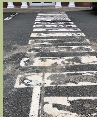
The surface of the route to Federal Street entrance is not stable or accessible.
