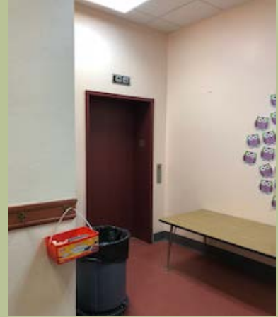
Long table and trash can is an obstruction to access the elevator at the Federal Street Elementary School.
