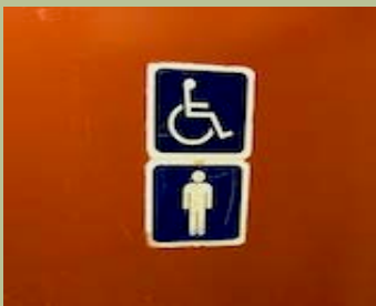
Accessible restrooms have non-compliant signage with no tactile characters in Federal Street Elementary School.
