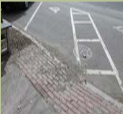
Accessible route from on-street parking location in front of 114 Main Street is uneven and not stable.
