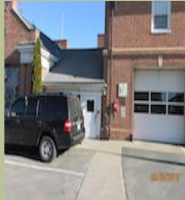
There is not an accessible route to the entrance of the fire station from accessible parking.
