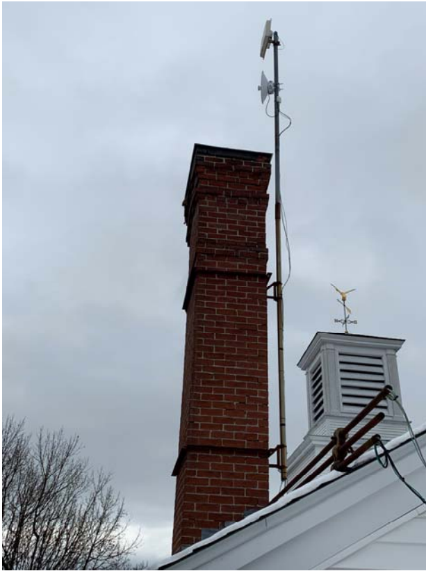
CHIMNEY AND MOUNTED IT EQUIPMENT
