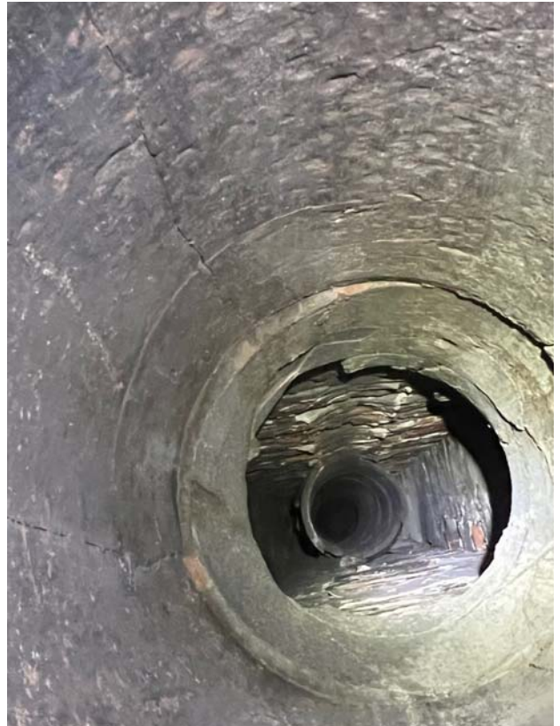
LOOKING UP FROM BOILER CONNECTION
