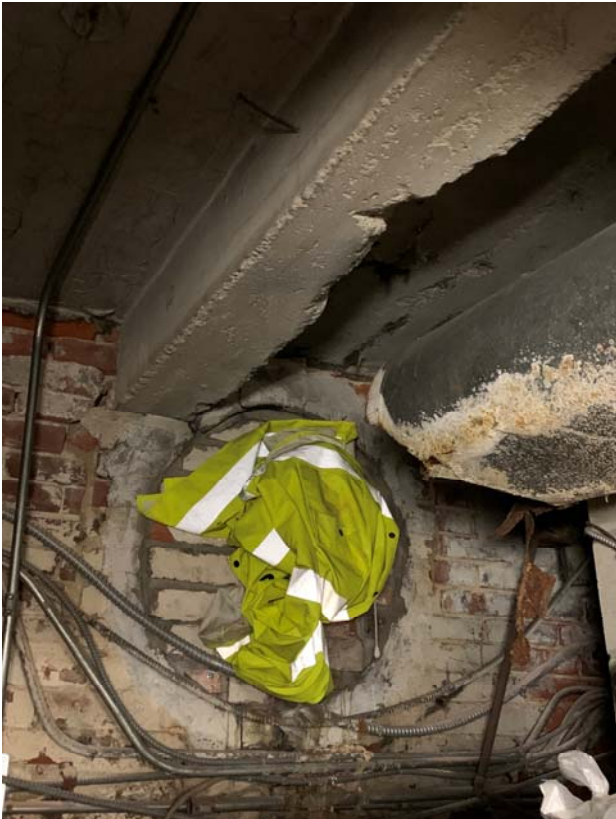
BASEMENT BOILER CONNECTION
