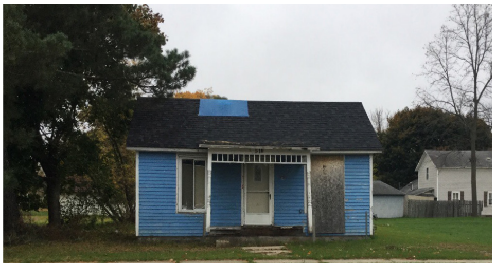
Example of poor housing stock
