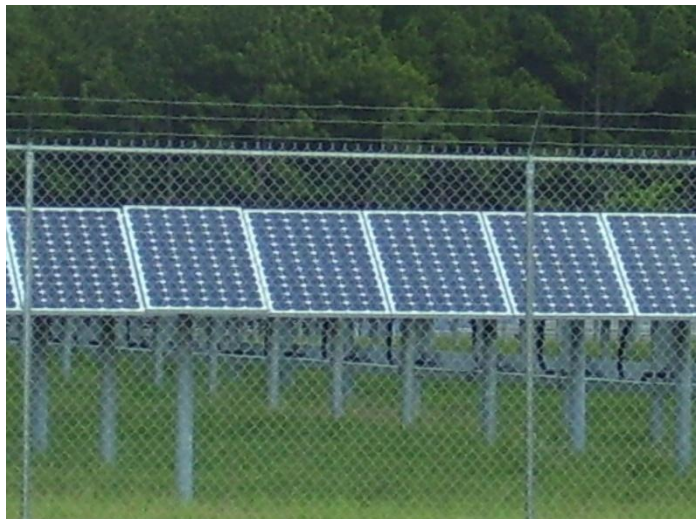
Solar Electric Panels at QVC
