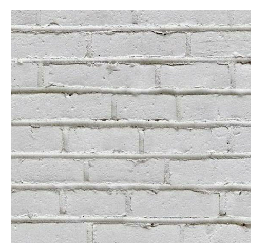
(EP-1) EXTERIOR GRADE WHITE PAINT OVER EXISTING BRICK FINISH ABOVE STOREFRONT AND ADJACENT EXTERIOR WALLS
