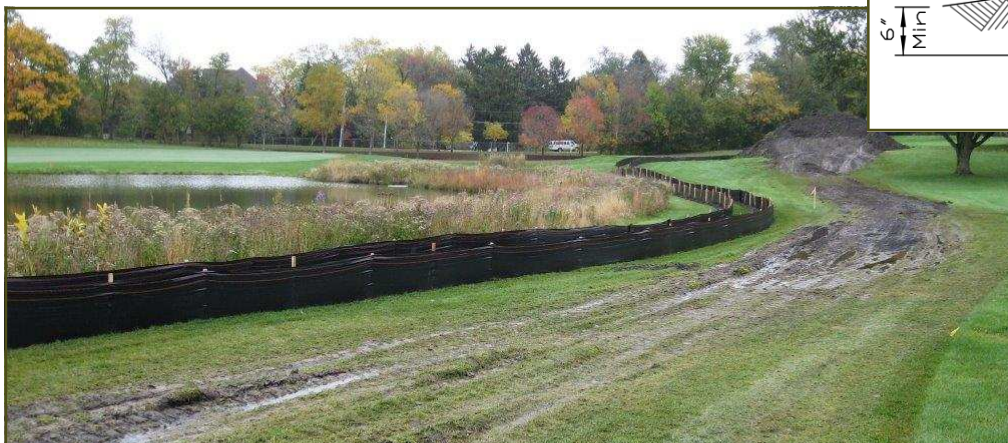
This is a real life example of a properly installed silt fence for the winter.
