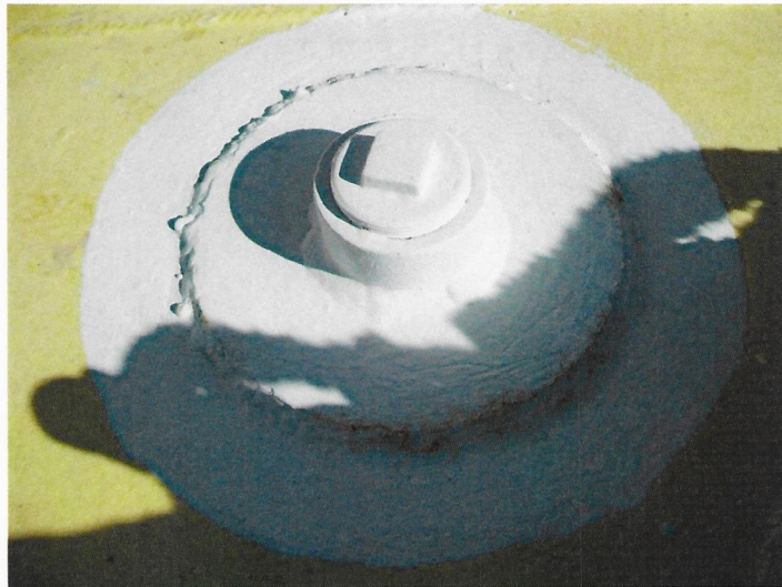
2) Roof rigging coupling not touched up with topcoat.
