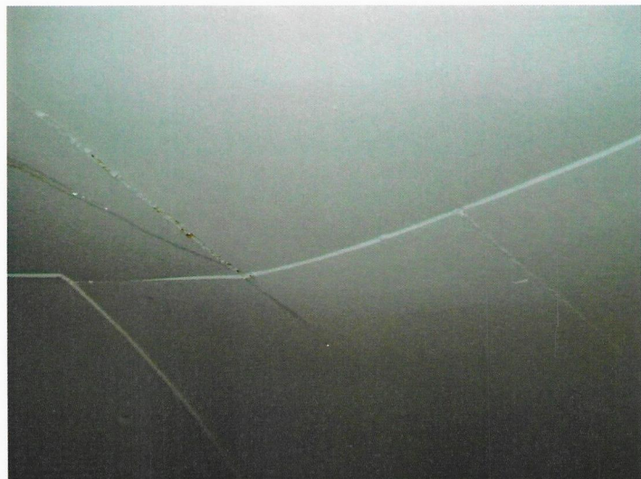
8) Rust bleedthrough on a roof weld seam.
