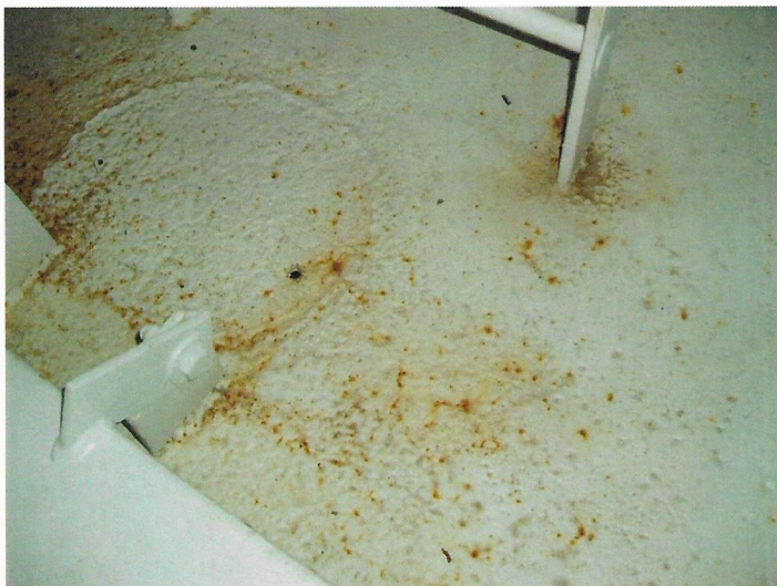
3) Steel grit rusting on top of the platform.
