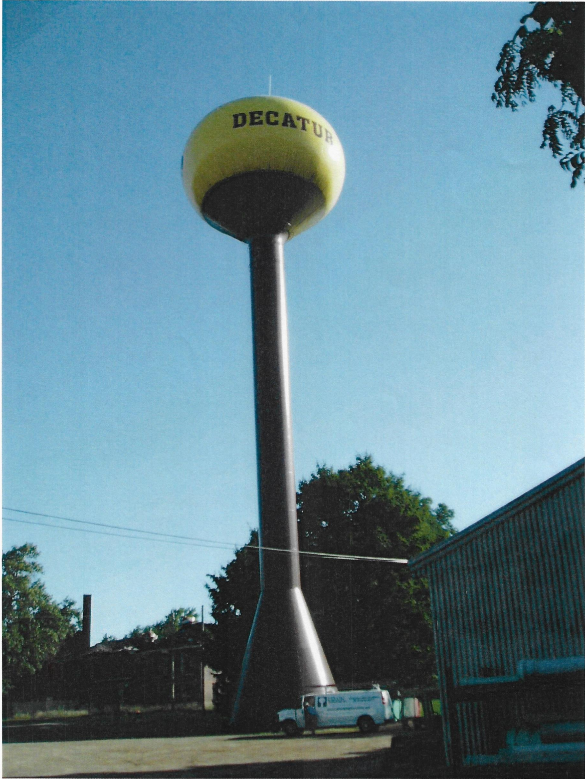
200,000 gallon spheroid water storage tank located in Decatur, Michigan.
