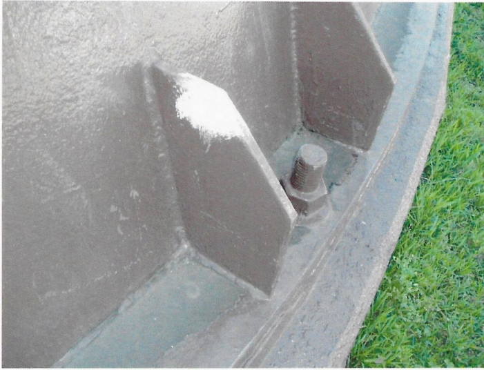
1) Ground attachment point not touched up with topcoat on anchor bolt chair.
