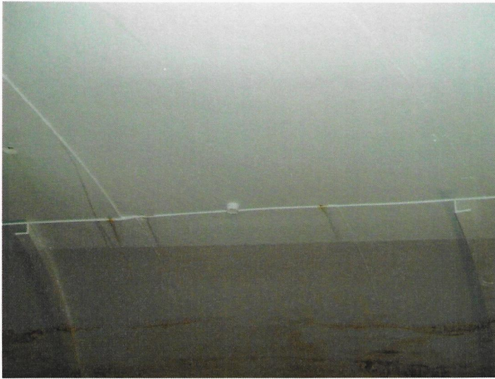
7) Rust staining on the caulked roof lap seam.
