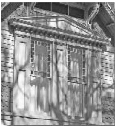
Free classic pediment and dentil band above two multi-lite windows. Small colored glass panes outline the upper lites of the 1-over-1 windows.
