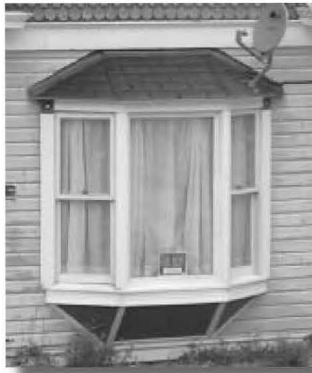
Beveled oriel bay window with half-hipped roof on side. Fixed, center window unit and 1-over-1 side units.
