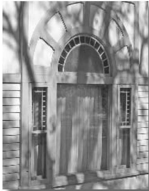
Tripartite (Palladian) window with a half moon window above the large middle unit. Small colored glass panes outline the upper lites of the side windows and the half-moon window.
