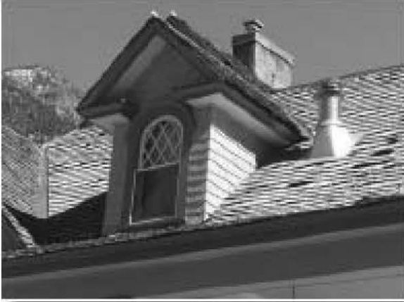
Pedimented dormer placed low on roof. Broken entablature return on pediment front, arched window with diamond-shaped lights and finial on pediment peak.
