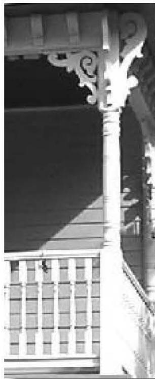
Turned spindlework columns with ornate multiple brackets. Turned balusters on railing. On Late Victorian dwelling.
