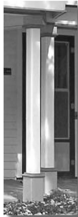
Square posts with square bases. No railing. On Dutch Colonial Revival style building.
