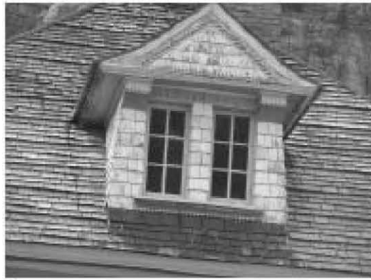
Pedimented double-window dormer. Entablature across pediment front, square shingles, and six-light windows.
