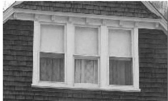
Group of three 1-over-1 windows in shingled gable with overhang and row of dentils above windows.
