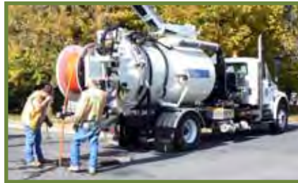
Town crews respond to sewer backup problems.
