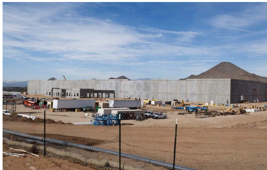
The 1.3-million-square-foot Big Lots distribution facility in Apple Valley will be largest in the High Desert. It will employ 300 construction jobs and up to 500 operational jobs when it opens in mid-2019.
