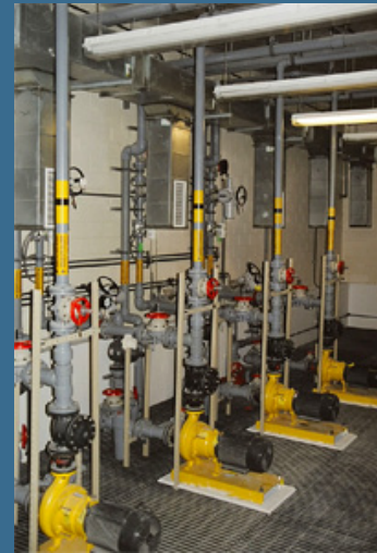
Disinfection dosing is the most challenging part of the treatment process since each storm brings a different loading of pollutants.
