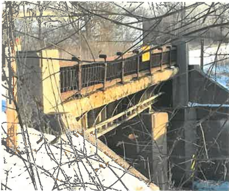
The railroad bridge over Ann Arbor Road is in need of repair, Plymouth Township officials insist. (Photo: Ed Wright | Hometownlife.com)
